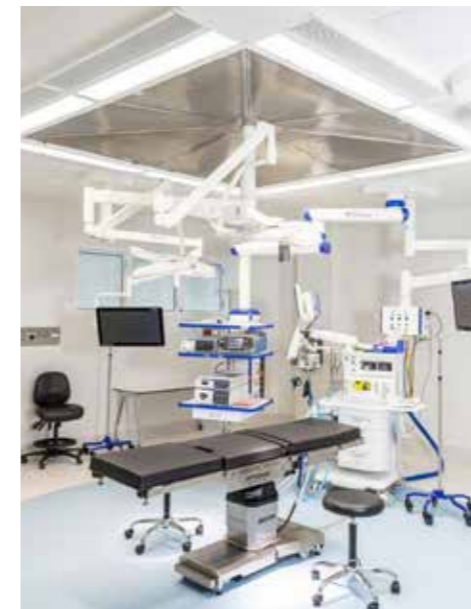
FOCUS 2000 installation, shown with integrated LED perimeter lighting, return air and central duct operating theatre light stem.
