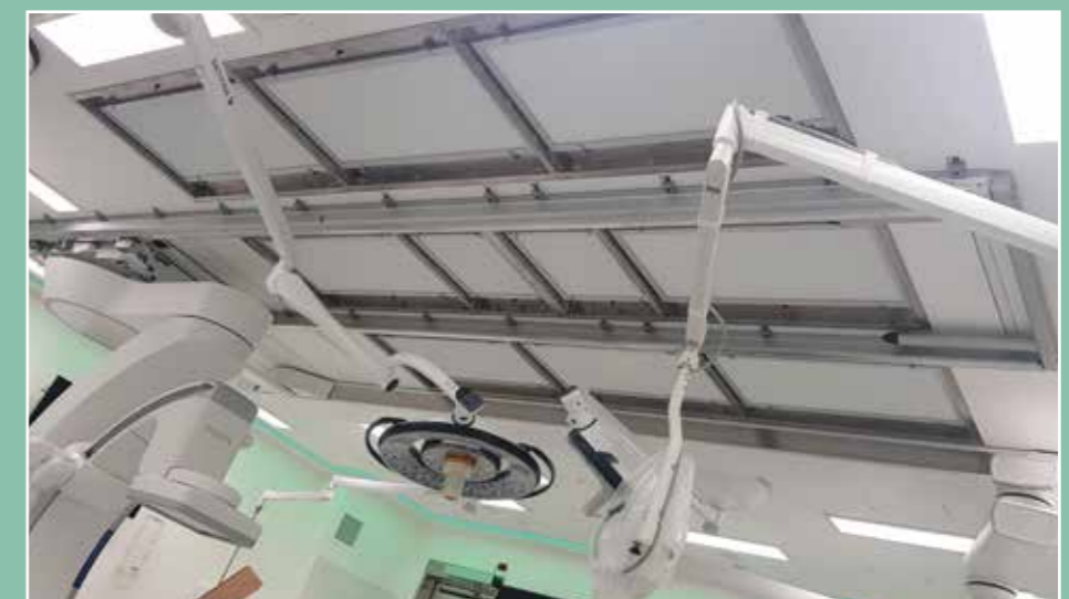
Hybrid FOCUS installations co-ordinated with medical imaging equipment gantry
